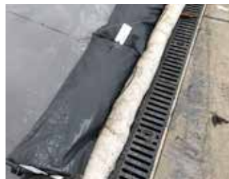
Stormwater Biochar Filter
